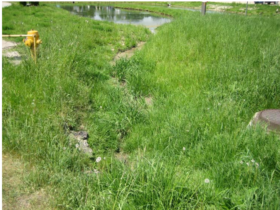
6. Offsite storm water management pond owned by adjacent property owner (Elmira Machine Industries) at low point in Martin's Lane on north side.
