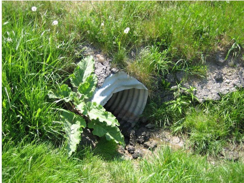
7. Culvert under Martin's Lane at low point where site discharge drains to.
